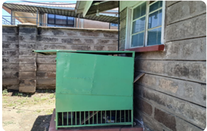
A photo showing a power backup generator at Lanet Health Centre. This was supported by county allocations and FIF funds.
